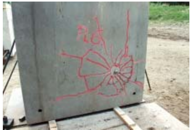
Figure D.8. Post test configuration for target 3 in test-series 1996:1. Back face of target plate 6.
