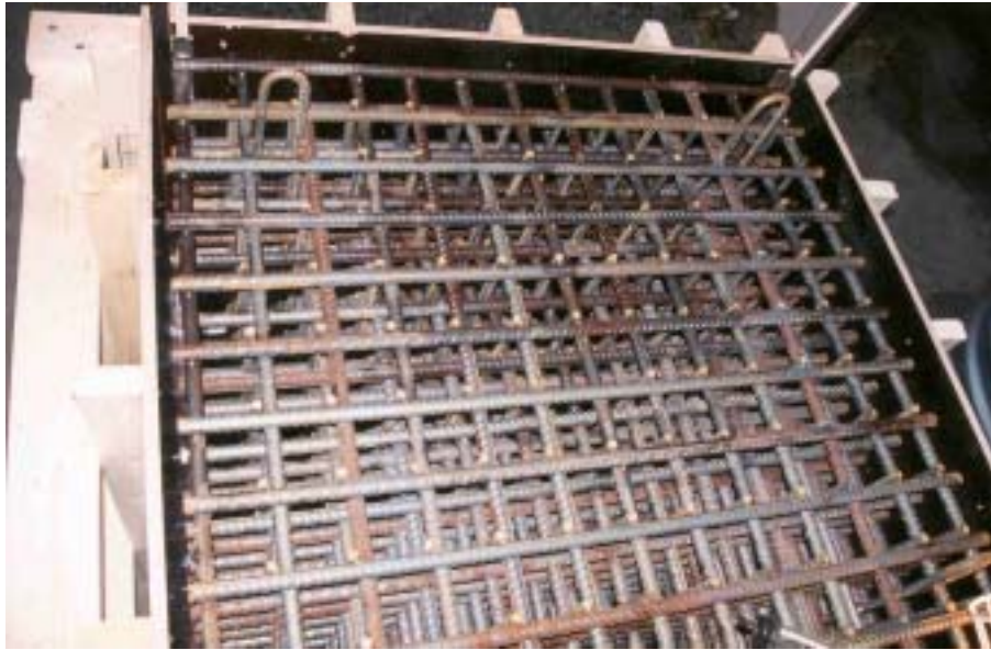
Figure 2.22 Target 7 of test series 1998:2. The reinforcement consisted of rebars ( \phi 32 mm) with a volume fraction of 6.5 %.
